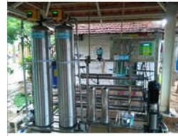
SS RO Plant
