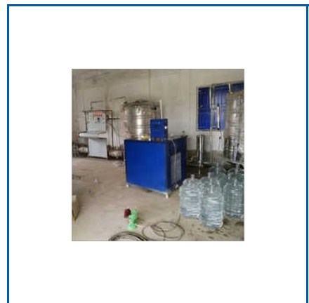
SEMI AUTOMATIC COMMERCIAL RO PLANT
