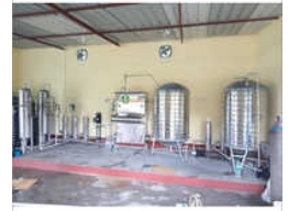
Packaged Drinking Water Plant
