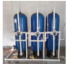
Industrial Water Treatment Plant
