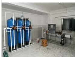
FRP RO Water Plant
