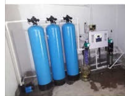
Industrial FRP RO Plant
