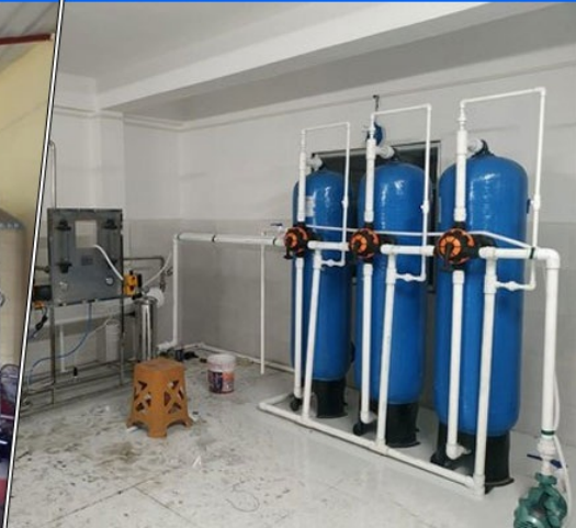
2000 LPH FRP RO WATER PLANT
