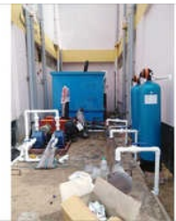
Industrial Sewage Treatment Plant
