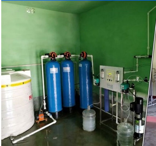
500 LPH SS RO PLANT
