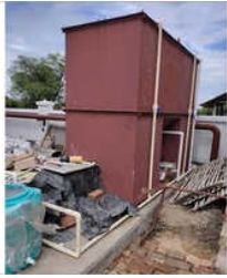
Industrial Effluent Treatment System
