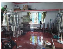
Automatic SS RO Plant
