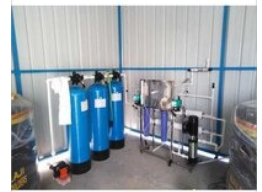
FRP RO Plant
