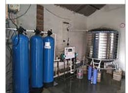
Water Filtration Plant
