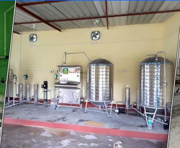
PACKAGED DRINKING WATER PLANT
